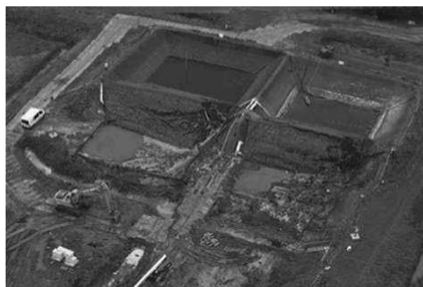
Figure 5. West and East dikes after failure.
