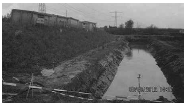
Figure 7. South dike during failure: fracturing of slope of ditch.
